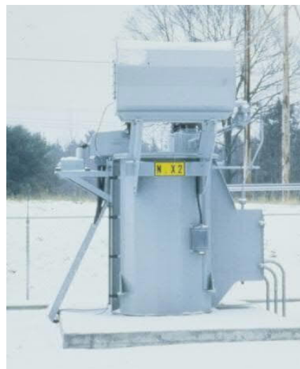
Plate 5.12 – Typical Auxiliary Power System Image: ©ABB
