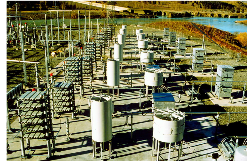
Plate 5.11 – Typical AC Switchyard Harmonic Filters Image: ©ABB
