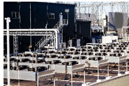
Plate 5.23 – Typical Outdoor Heat exchangers Image: ©GE
