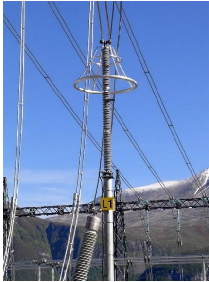
Plate 5.7 – Typical HV Surge Arresters Image: ©ABB
