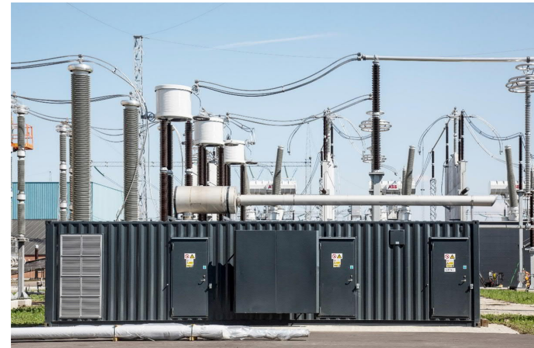
Plate 5.13 – Typical Diesel Generator Image: ©ABB
