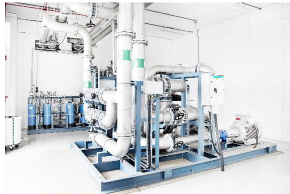
Plate 5.22 – Typical Water Pumping Station Image: ©ABB
