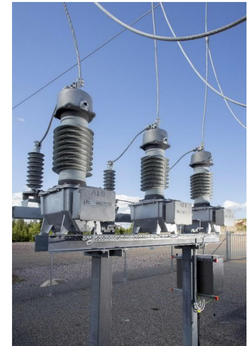
Plate 5.16 - Typical Voltage Transformer Image: ©ABB
