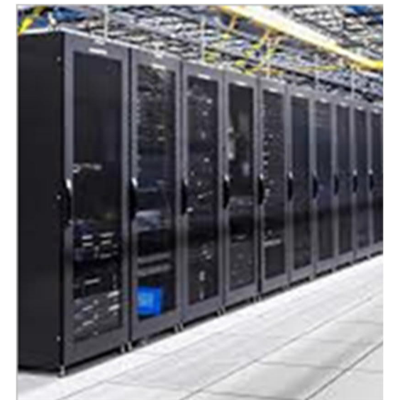
Plate 5.38 – Typical cabinets (Copyright – B&M FOC Review Report Issue D Sept. 2018)
